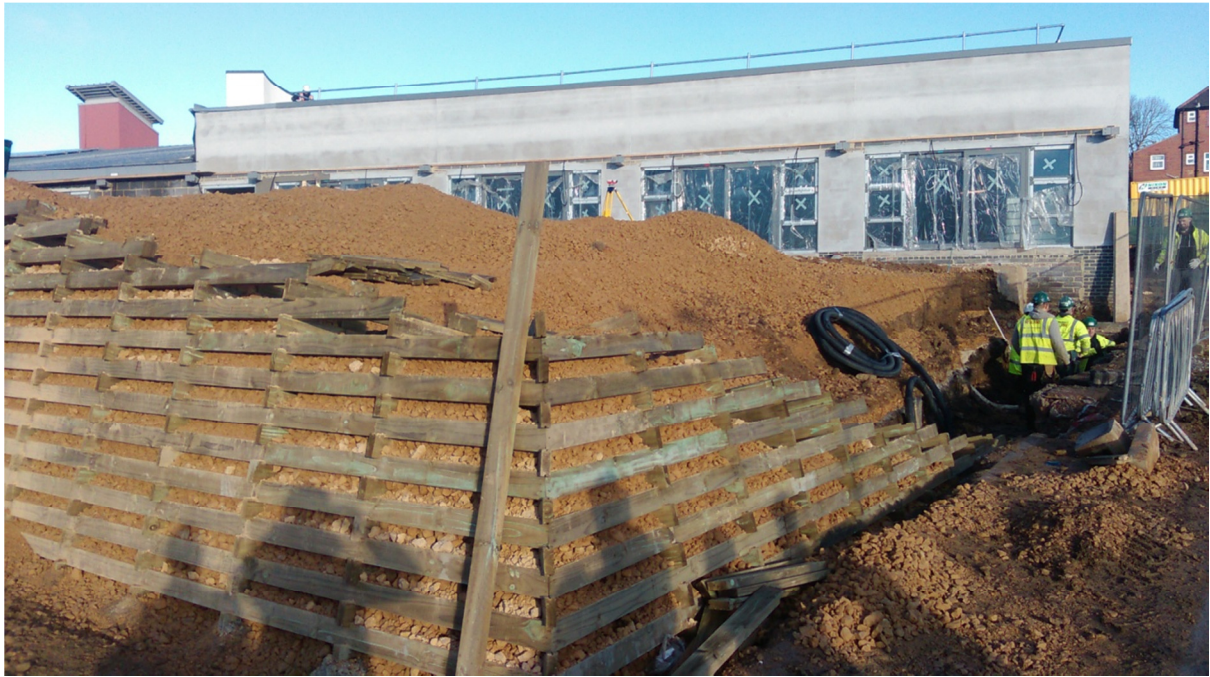
The crib wall for the new raised playing area for our 0-3 setting.
